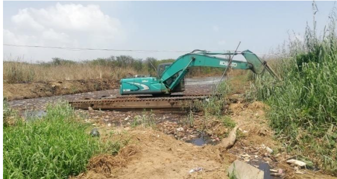
Figure 9: Canal which connect to the dumping site and stay as stagnant with full of garbage
