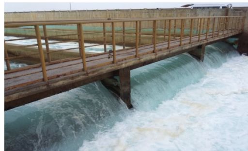
Cooling water outlet tank
